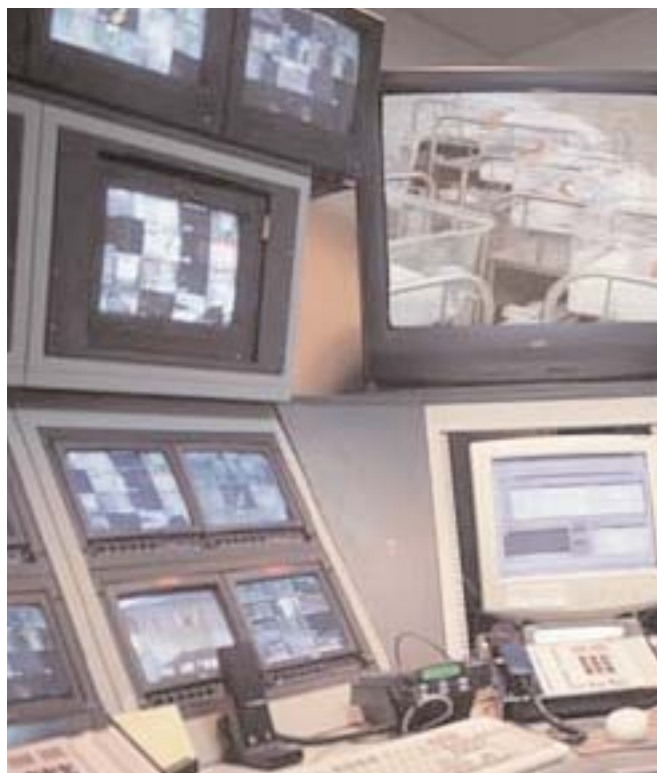
One of the areas covered by NFPA 731 is closed circuit TV (CCTV) and video surveillance systems.
